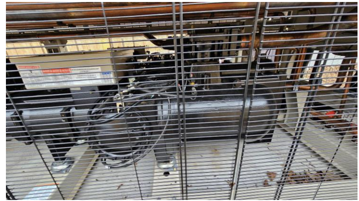
Lowell ES Chiller Compressor
